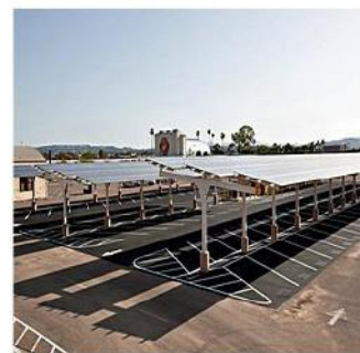
PVs can also be mounted on the ground or auxiliary structures. These collectors provide shade for parked cars at MCAS Miramar. Photo Credit: MCAS Miramar
