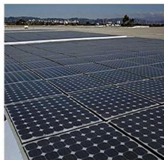
PV system on a mail processing center in Los Angeles. PVs are one of the most reliable renewable energy technologies, and building integration can be straightforward. Photo Credit: Bill Calma
